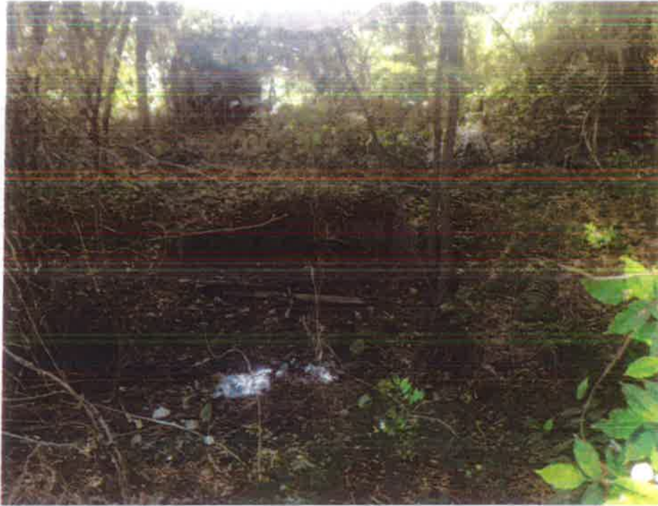
Figure 4-South Drainage Basin - 30" CMP just upstream of Speedy Wok
